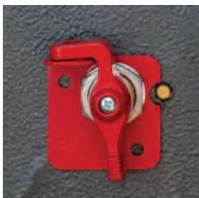
Isolation switch in OFF position
