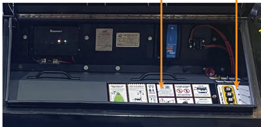
Inside hydraulics & control panel compartment
