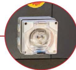
Figure 8a Battery Charger socket 240v
